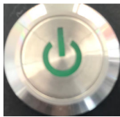
Fig. 11: Main battery switch not pressed
